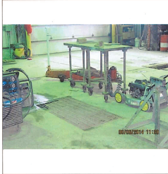
IMG_0253 (Small).jpg Drain de plancher.
